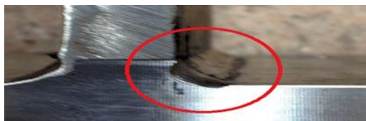
Small weld Bead
